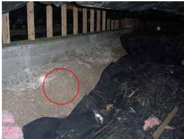
Photo 9 bare earth, vapor barrier moved
