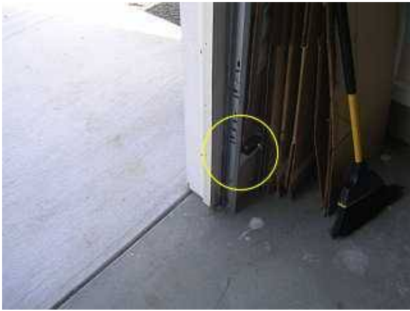
Photo 6 Recommend lowering to 4-6" for safety
