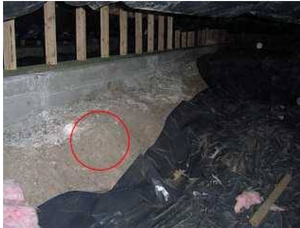
Photo 9 bare earth, vapor barrier moved
